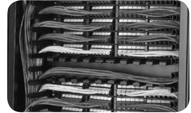
Glide Cable Manager shown in cabinet
